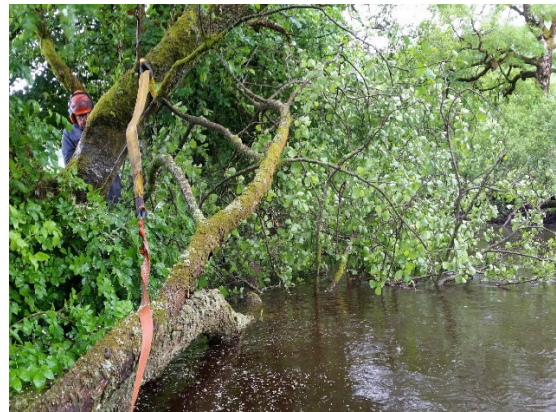
Fig. 2.2 Felled trees were winched into the bank to provide cover for fish
