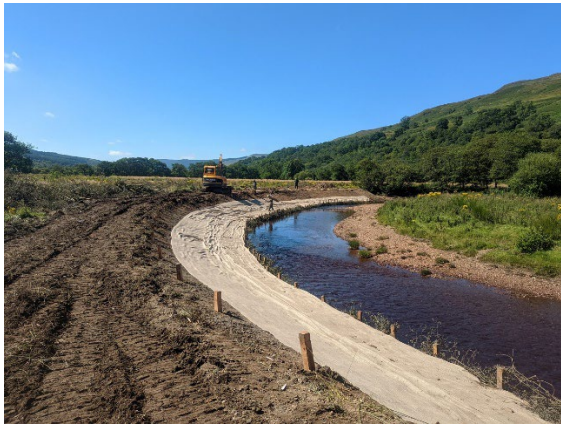
Fig. 2.11 Hessian layer installed to aid bank recovery and securing posts driven into the top of the bank
