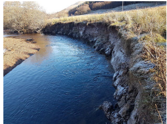
Fig. 5.4 Bank erosion & collapse (site B3b)
