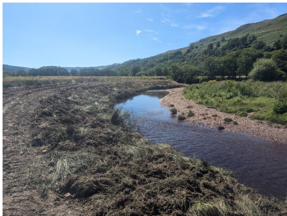
Fig. 2.13 The turf laid onto the willow secured by a fencing wire lattice.
