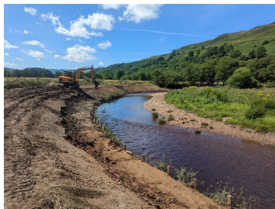
Fig. 2.10 Track machine securing the bank behind the brush to protect the new bank
